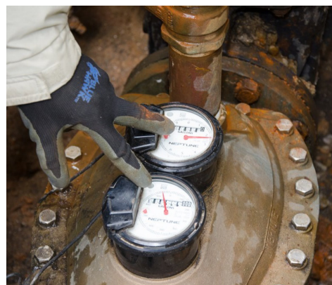
Figure 10 Checking the Register Dials
