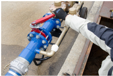
Figure 25 Back-flushing the Meter
