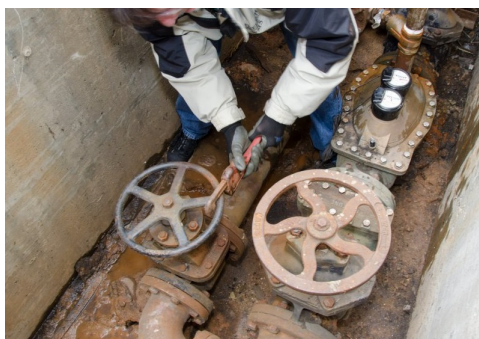
Figure 9 Opening the Bypass Valve
